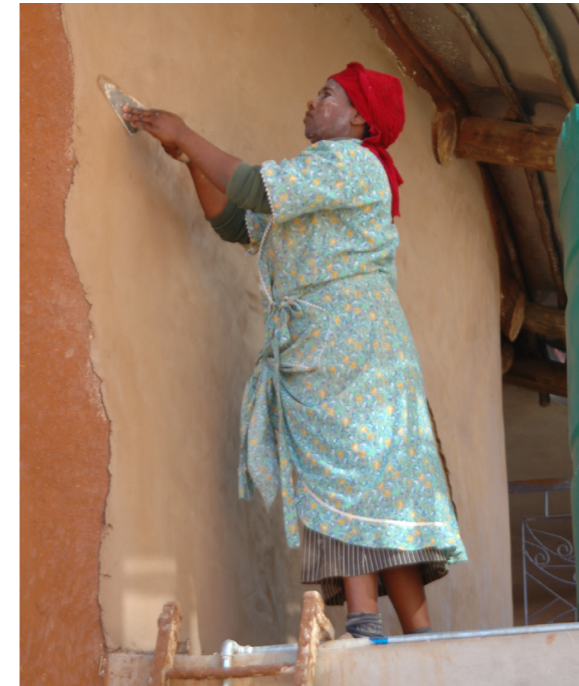
Lime-sand plaster with fresco finish at 7 Fountains Primary School, Kokstad, KwaZulu-Natal
